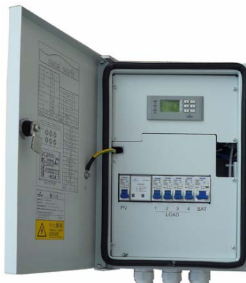
Figure B.7: Energy controller
