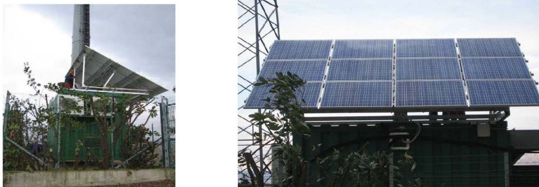
Figure A.2: Installation of PV panels above shelters (with positive shadowing effect on equipment)
