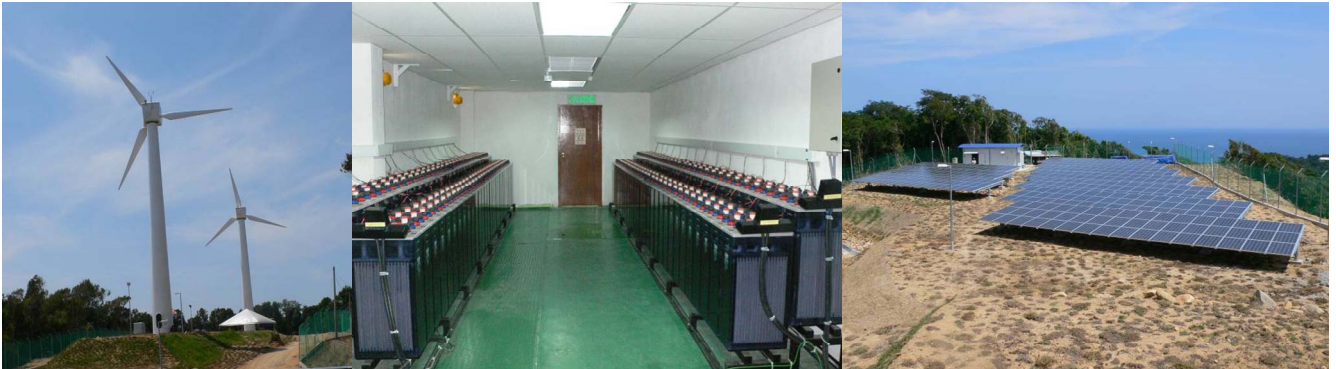
Figure 10: Lead-acid battery installation in a 500 kW renewable sources power plant with combined eolic and photovoltaic generation
