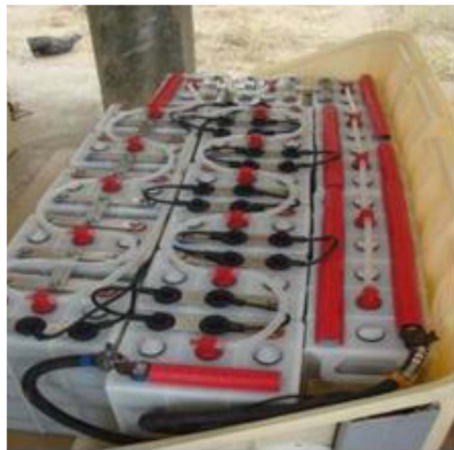
Figure A.6: Example of a NiCd battery in an African country
