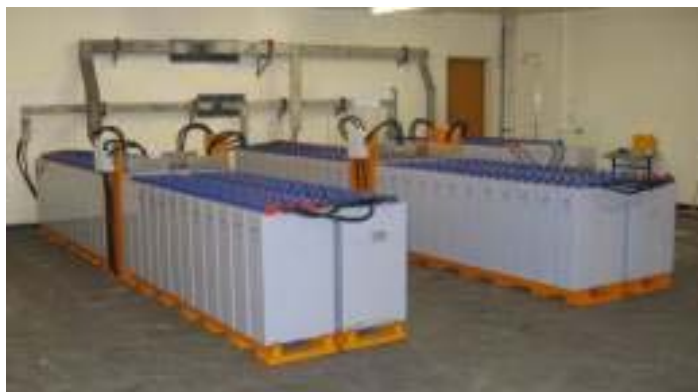
Figure A.1: 48 V multistring lead-acid battery in a telecom centre
