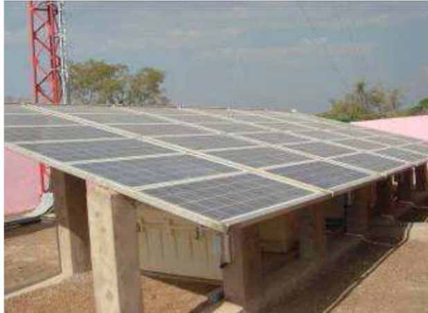
Figure A.5: Example of a solar power system for a radio mobile base station equipped with solar system equipped with flooded tubular lead-acid battery referred to as OPZS
