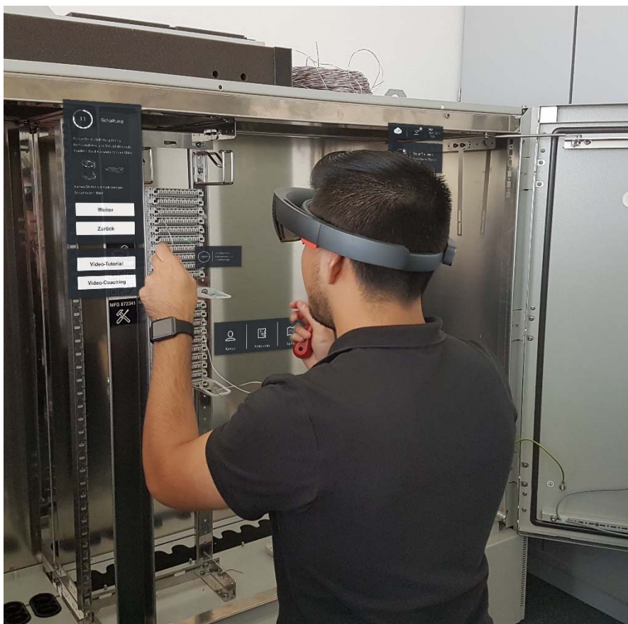
Figure 16: Wiring inside a switching unit
