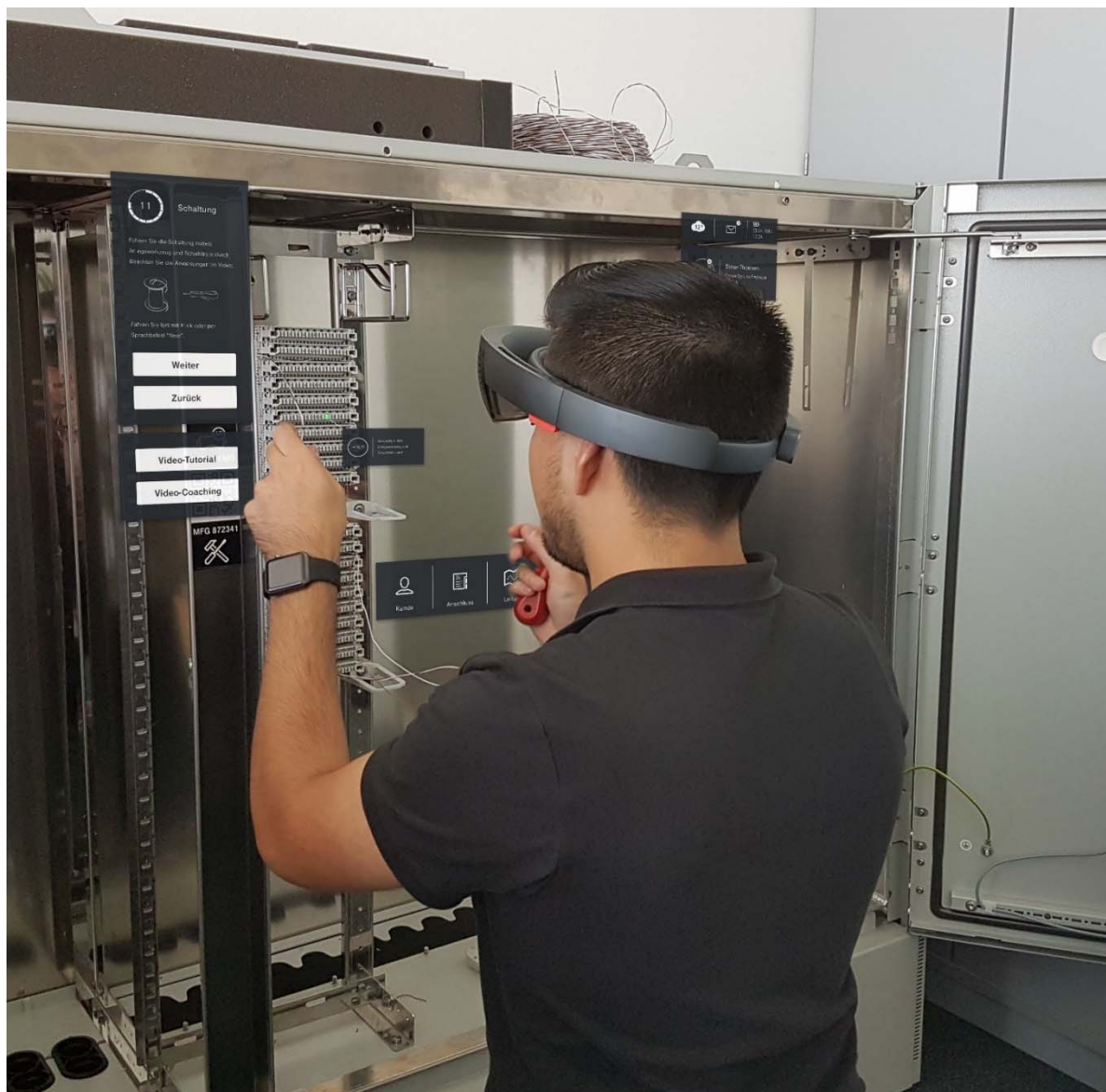
Figure 5: Wiring in a street cabinet
